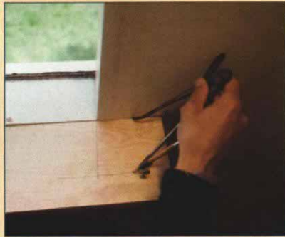
Fitting a window stool. The author uses a combination square to mark the outside corner of the window opening on the stool (top photo above). Then he uses a bevel square to measure the angle between the window jamb and the front edge of the stool. This angle is scribed on the stool through the corner point (middle photo above). Finally, he sets his pencil compass to span the distance between the corner of the opening and the corner mark on the stool, then scribes the stool's horn to the wall (bottom photo to above).
